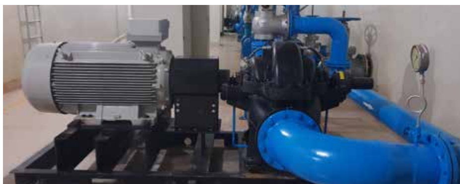
NR. 2 SKDZ-4P 200-630 400kW VIETNAM HYDRAULIC POWER STATION
