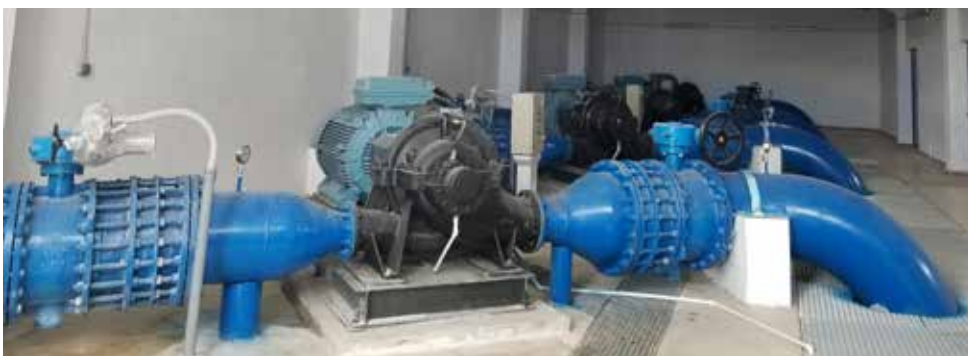
NR. 4 SKDZ-4P 200-630 400kW ALGERIA DRINKING WATER SUPPLY
